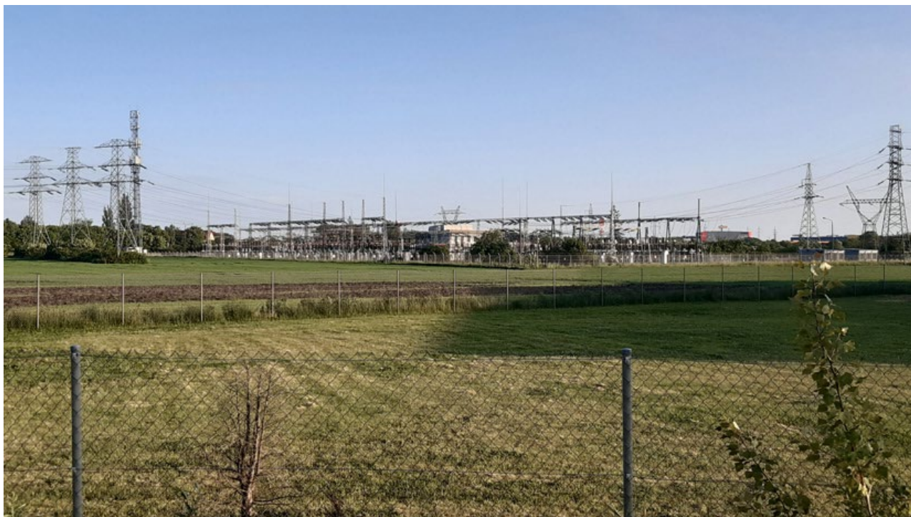
III. 7. Klecina wedge: Transformer station: the Main Power Supply Point "Klecina" R-1. Photo by J. Rubaszek.
