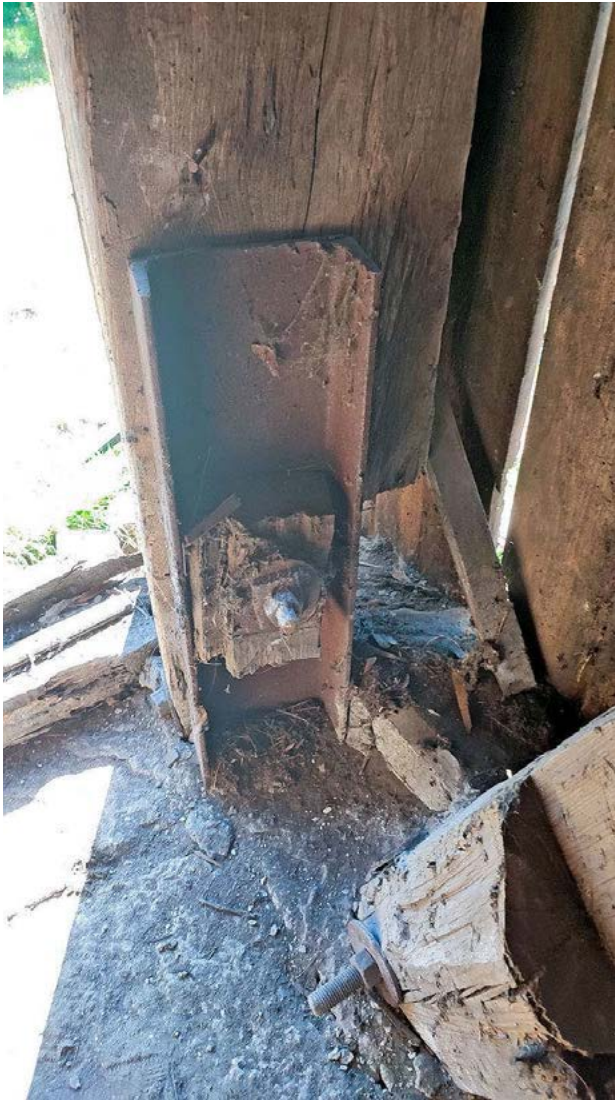
Ill. 11. The existing condition of the lower sections of the posts indicates that no joint replacement was carried out. Measures were limited to cutting off the lower parts of the posts and setting new foundations with joints using vertical channels. Original photo, 2023.
