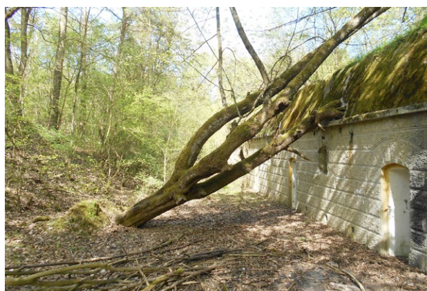
Ill. 6. Windthrow leaning on a shelter at Fort Parski in Grudziądz, 2018. Photo by the authors.
